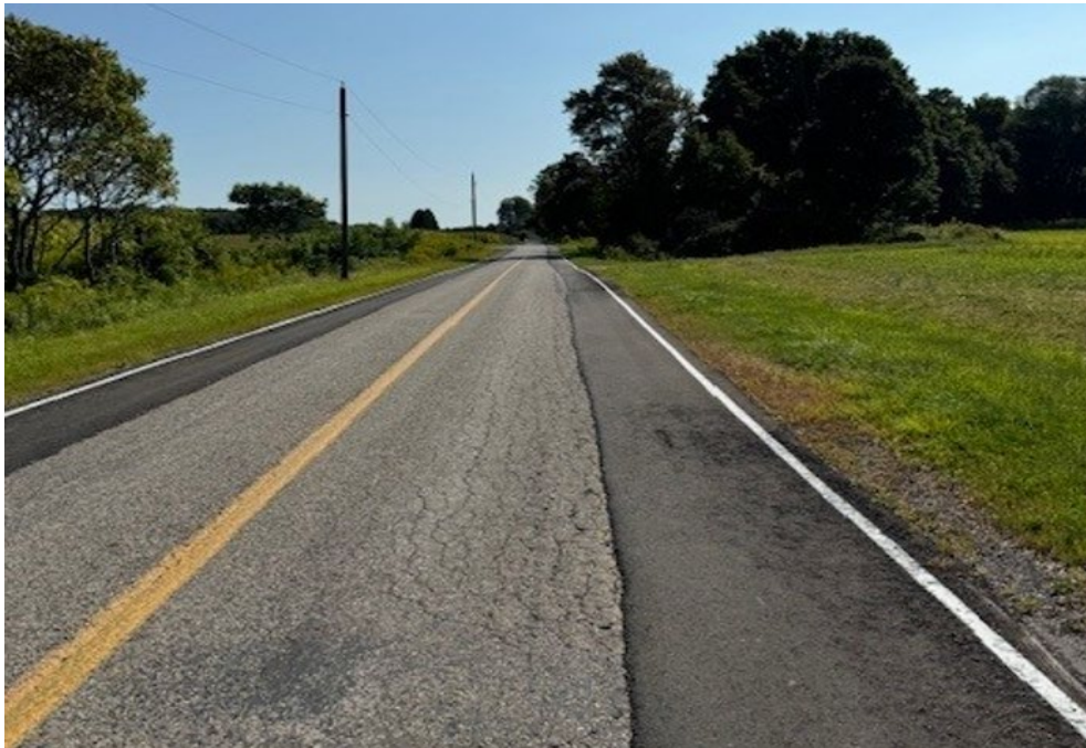
Substandard Ditching - Scotch Line west of Coon Road
