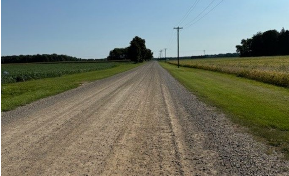
Substandard Ditching - Scotch Line west of Boxall Road
