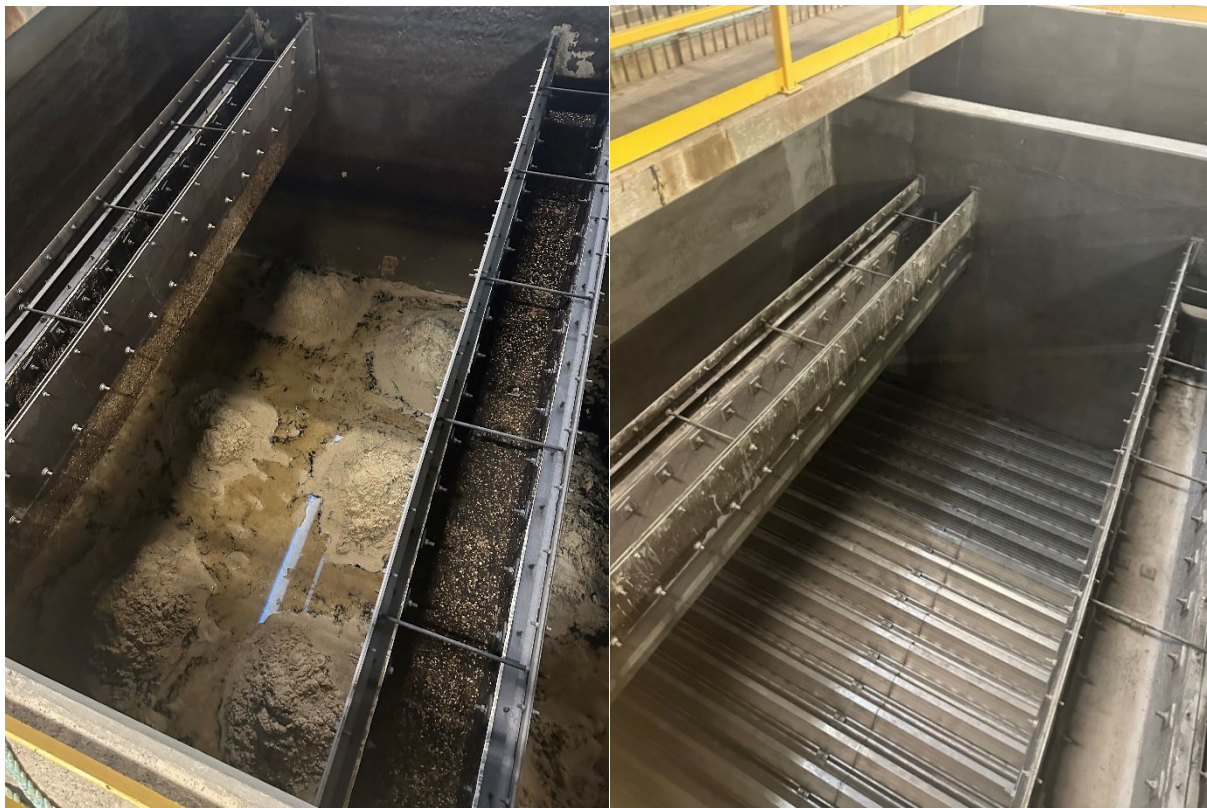
Figure 6a: Filter #3 pre-repair. The filter media (anthracite and sand) and underdrains have been removed to perform repairs. The filter media (sand) that is present on the concrete filter base confirms leakage between the underdrains and the concrete base.
