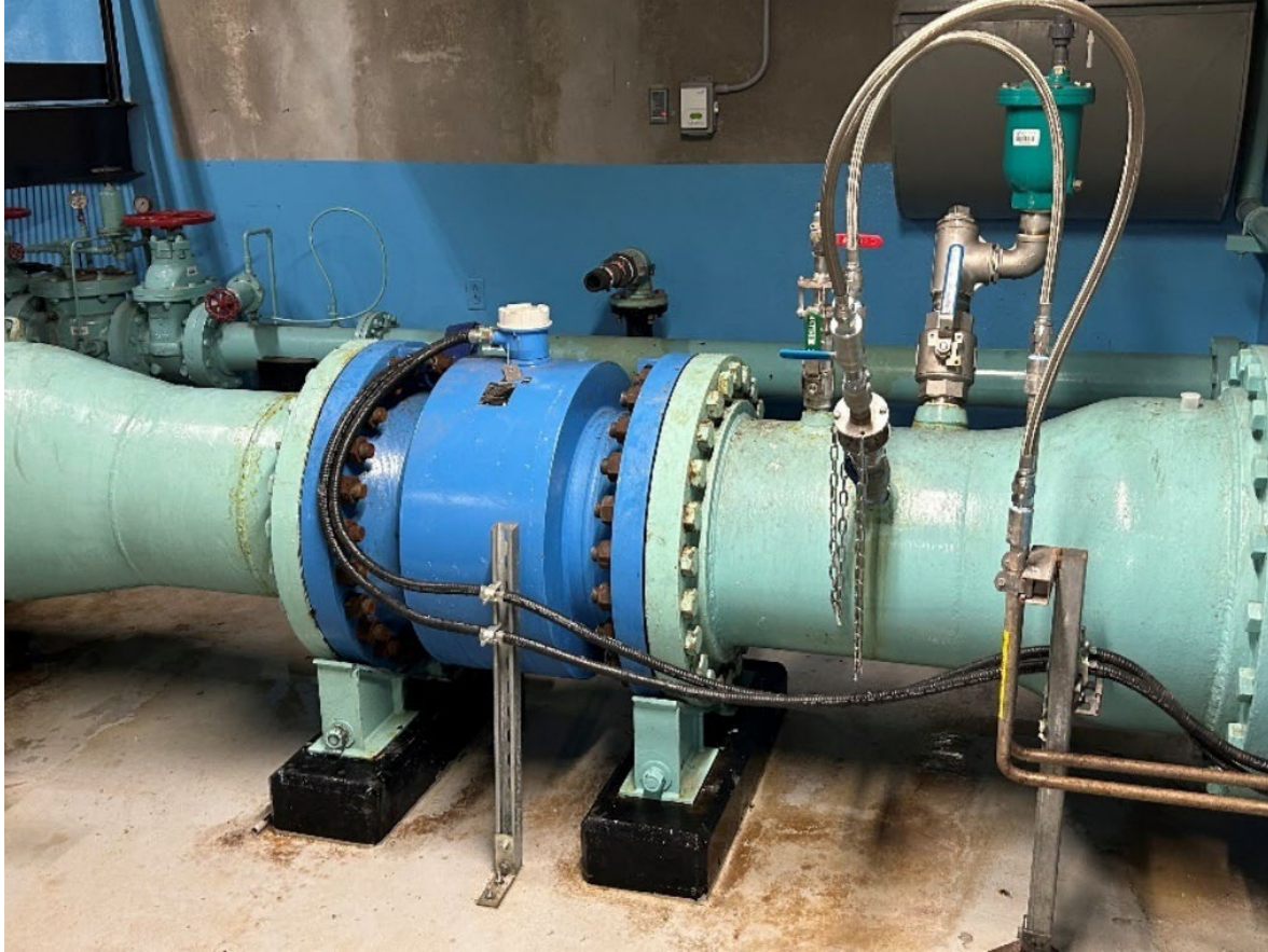
Figure 8: Completed modifications to the sodium hydroxide injection system on the west treated water discharge header.
