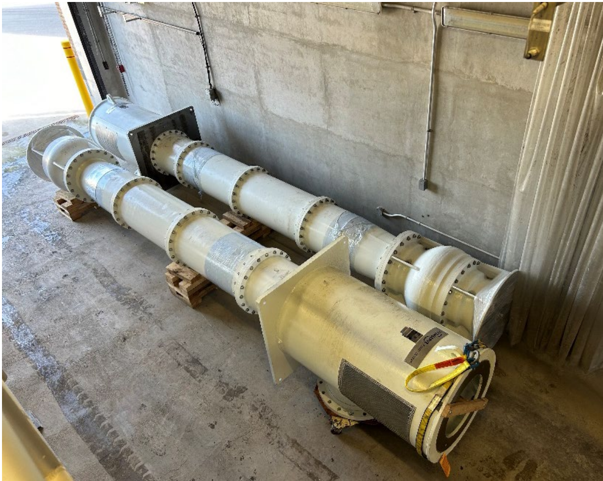
Figure 5: The new pumps delivered to the Elgin Area WTP in October 2024.
